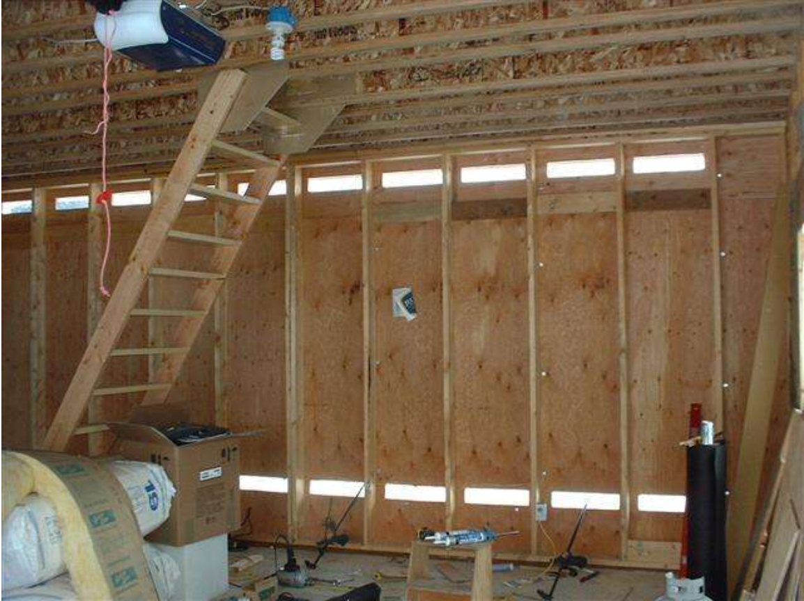
Figure: Collector entry and exit vents from inside barn
