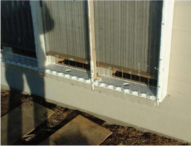
Figure: Lower sill with summer vent holes – lower vent and absorber screen support are visible above the sill.
